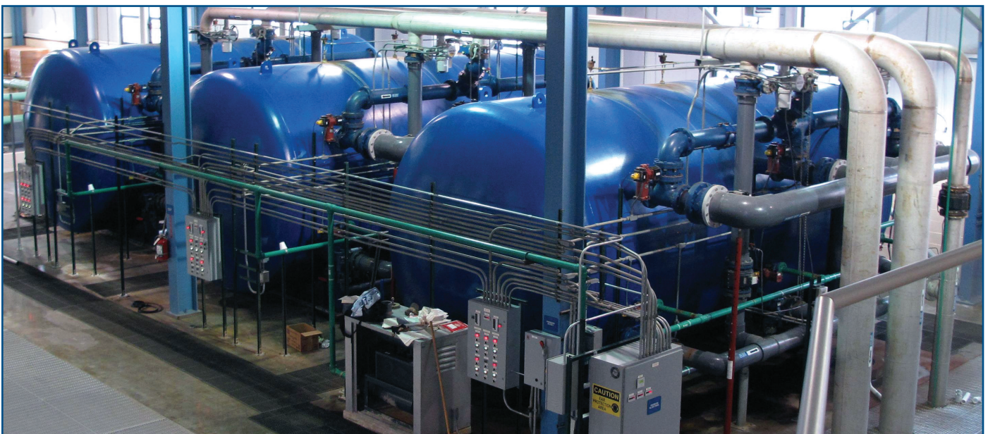
GreensandPlus Pretreatment for RO Filter System 4.2MGD
