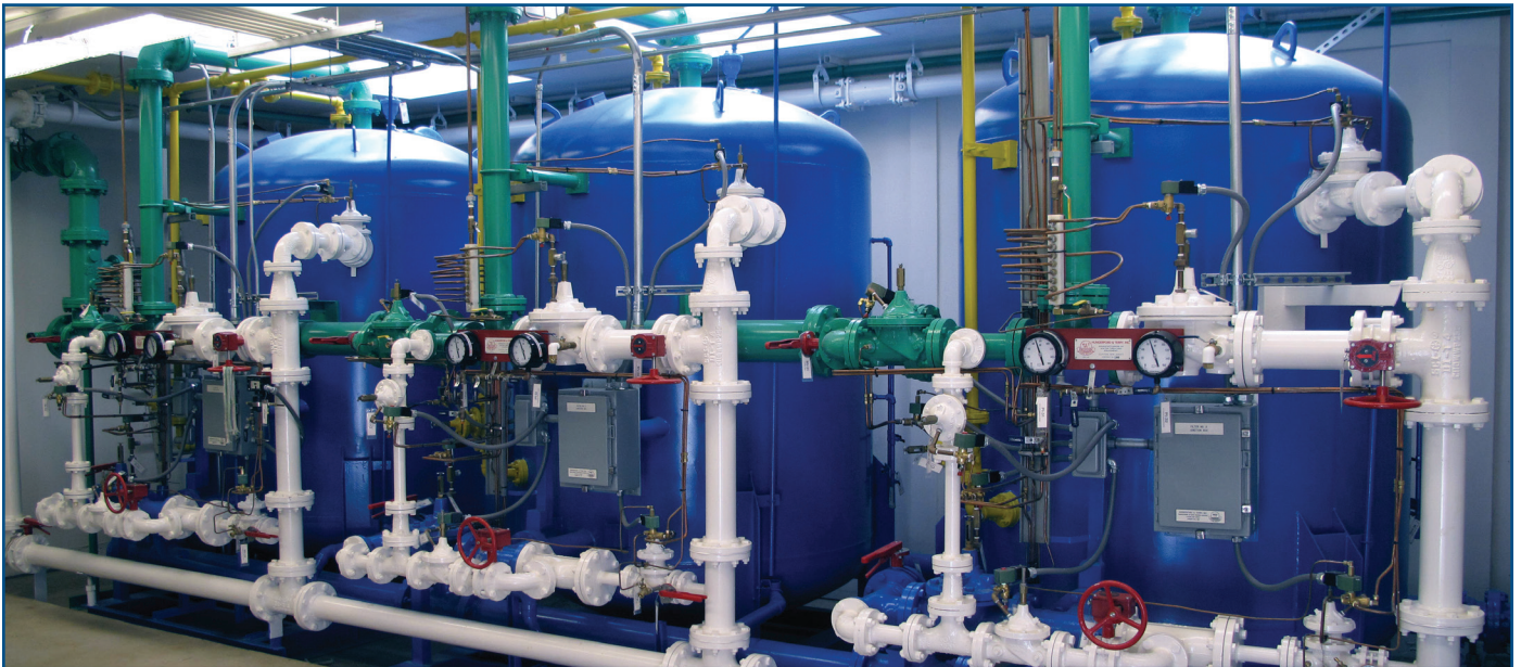
This is an example of the 1.5 MGD municipal filter installation with air/water wash, by Hungerford & Terry.
